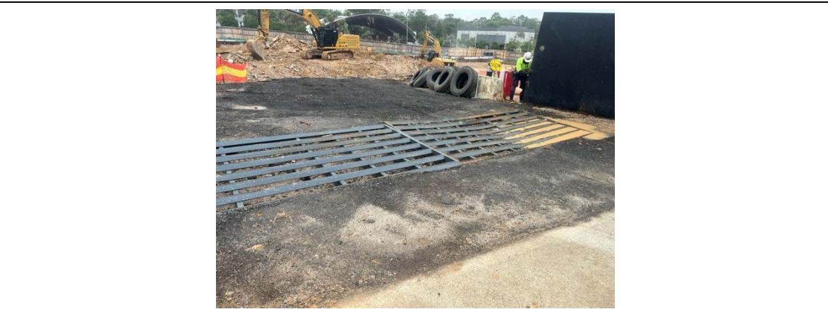
Photo 9: Shaker grid in place at heavy vehicle exit onto De Clambe Drive. No tracking observed.
