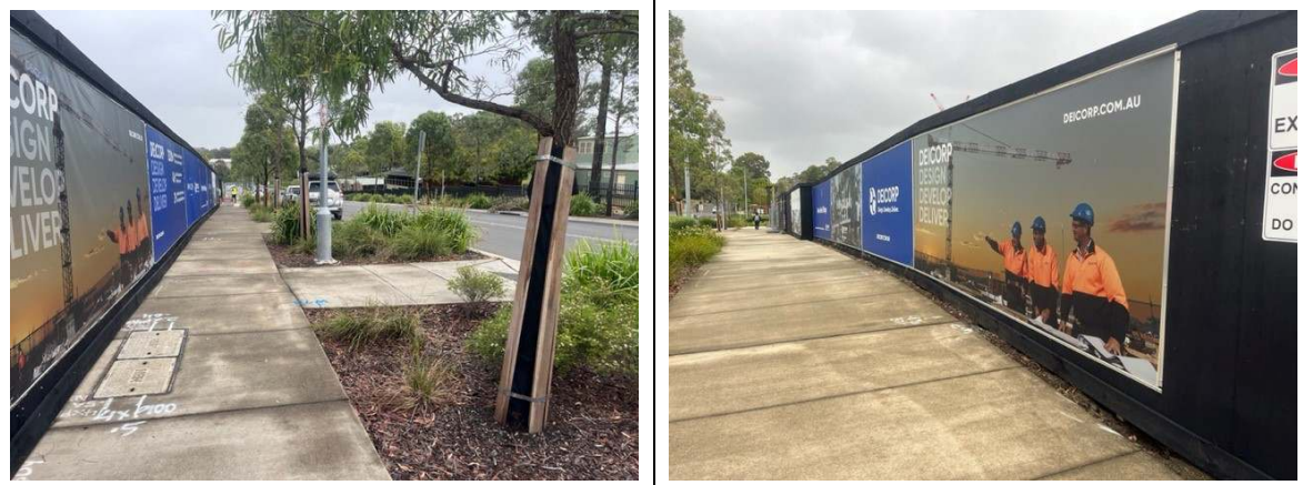
Photos 7&8: Hoarding in place along site boundaries. Tree protection in place on De Clambe Drive.
