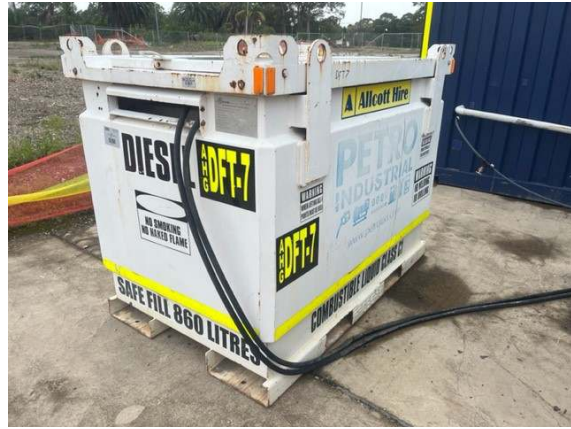
Photo 17: Diesel fuel cell on hardstand in the site compound
